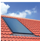
Clearline Solar heating panels
