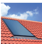
Clearline Solar heating panels
